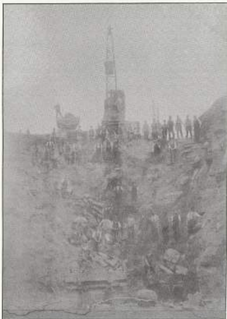
Plate 1. Workers engaged in the excavation of Winterbourne Down railway cutting circa 1902. The line was opened for passenger traffic on 1st July 1903.
